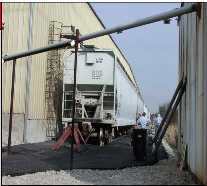
Unloading staff shown above at Silgan Plastics Corporation are busy placing the finishing touches on their railcar unloading facility which was recently upgraded.
