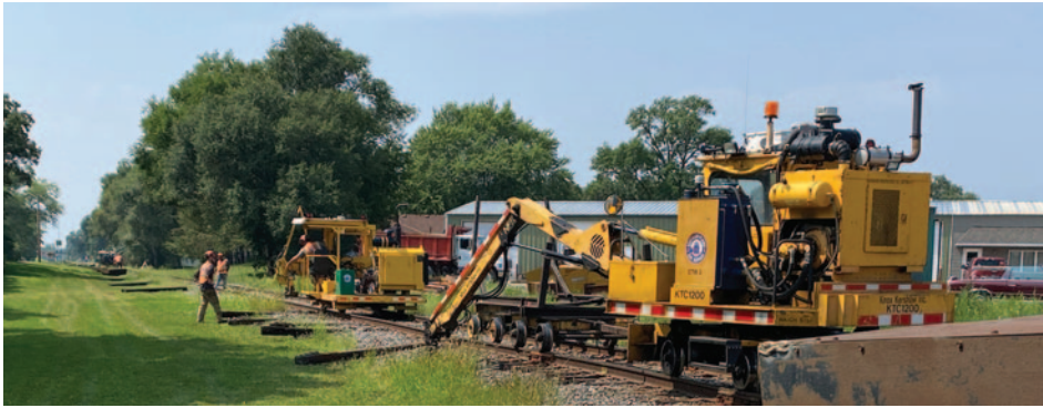
Our work crew renewed track in August as part of the Minnesota Rail Service Improvement grant.
